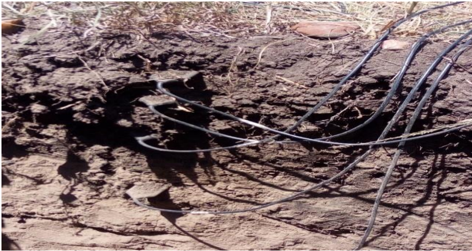
Fig. 4. Installed 5TM-ECH 2 O Soil Moisture and Temperature Capacitance probes
