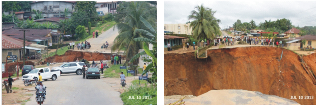
Figure 1. A section of the road destroyed by an impressive gully channel
