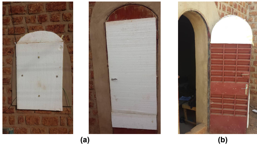
Fig. 5. Image showing (a) window insulated with polystyrene; (b) Insulation of door with polystyrene.
